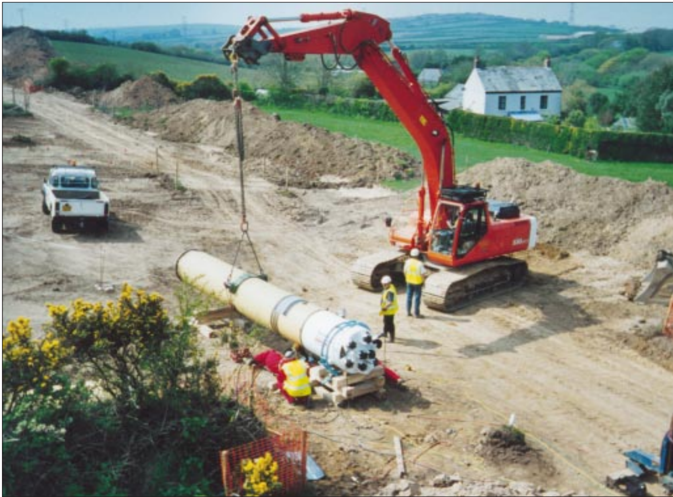
Photograph Above. Setting up for the 1 st Rock Bore which turned out to be an unprecedented success.
